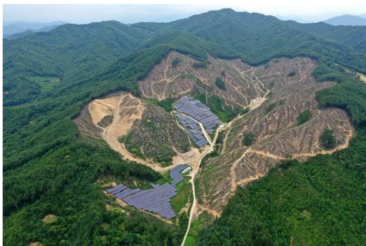
A solar power plant built in the mountain area, Jangsu-gun, Jeollabuk-do (Source: The Hankook Ilbo)
